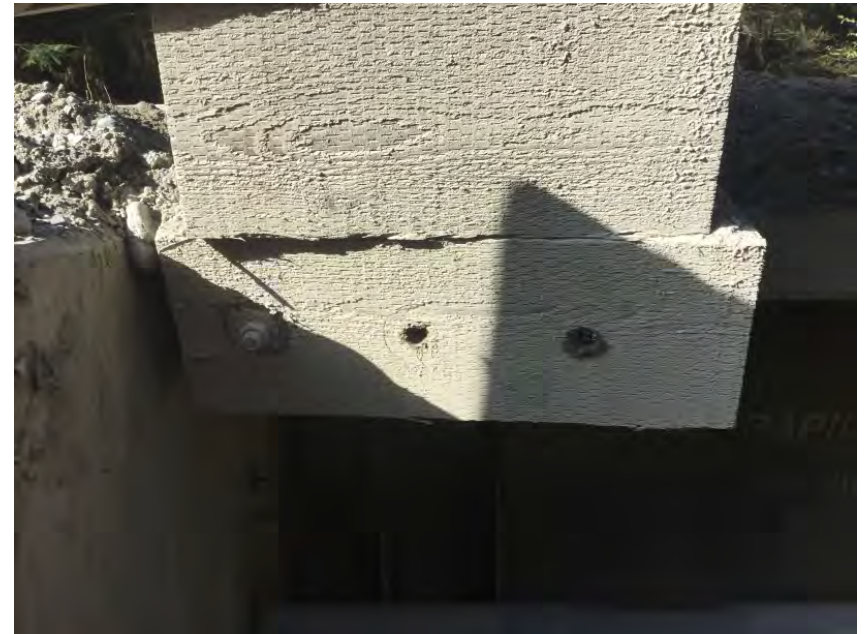
Side block bolts missing on damaged guardrail
