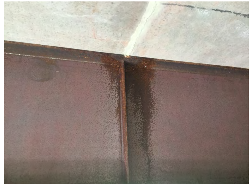
Evidence of water getting through deck joints
