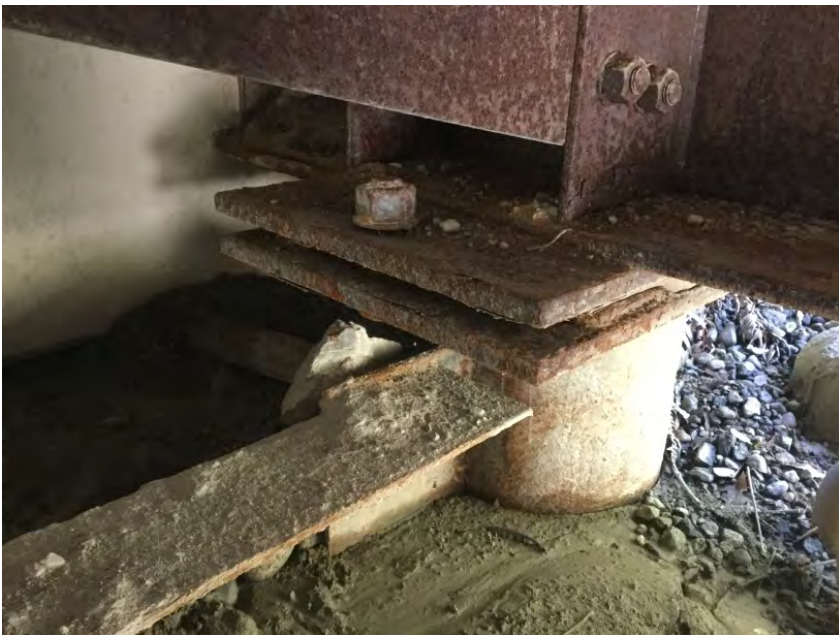
Minor corrosion noted on bearings
