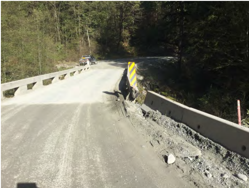
Damage to downstream right approach guardrail
